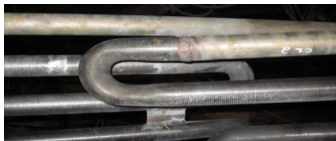
Figure 2: Colmonoy 88 Spray & Fuse overlay protecting Inconel tubes in core of Super heater boiler [4]
